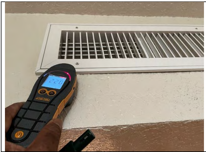
37. View of elevated moisture levels using Protimeter around supply diffuser in PEI 345
