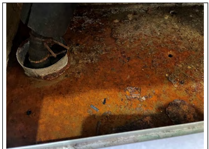
42. View of standing water in HVAC return box likely caused by drip pan out of alignment
