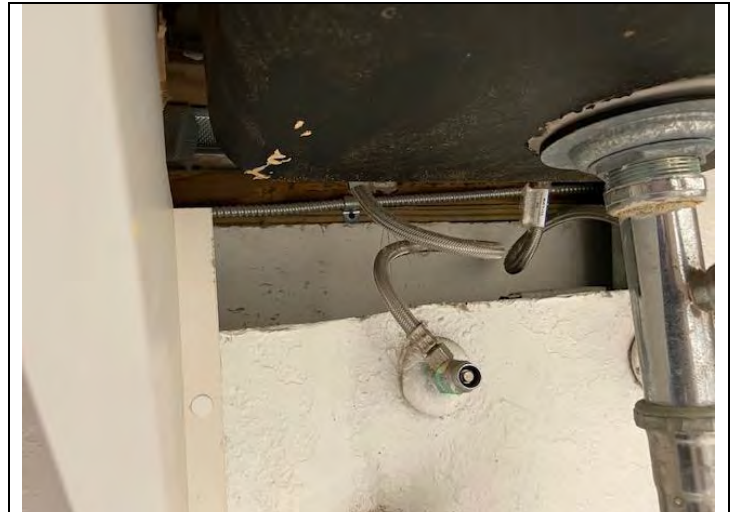
16. View of SVG under sink in PEI 232
