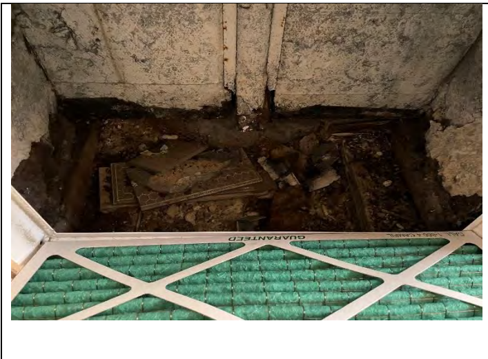
35. View of broken HVAC return box with visible debris in PEI 317
