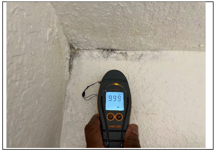
14. View of SVG and elevated moisture levels using Protimeter on restroom ceiling PEI 223
