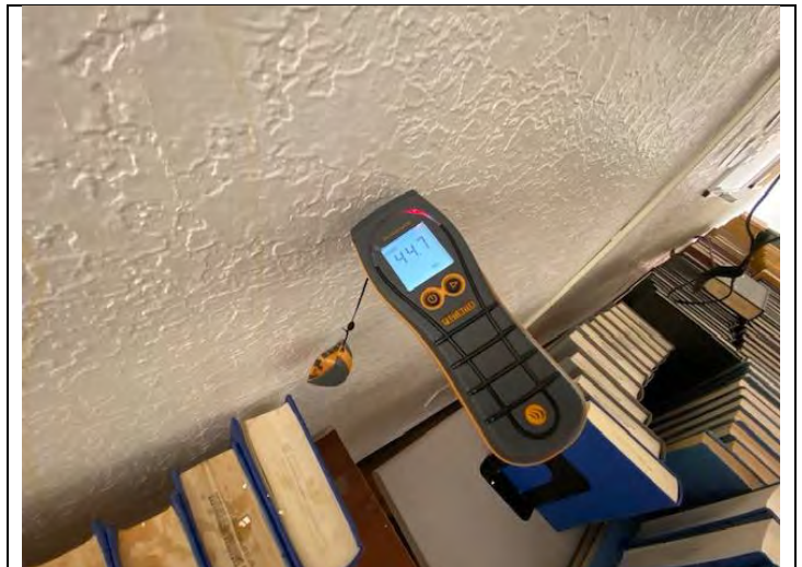
24. View of elevated moisture using Protimeter on south wall in PEI 2 Lounge
