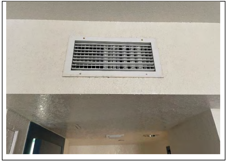
8. View of condensate on supply diffuser in PEI 216
