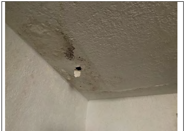
22. Close up view of SVG on ceiling outside restroom in PEI 2 Lounge
