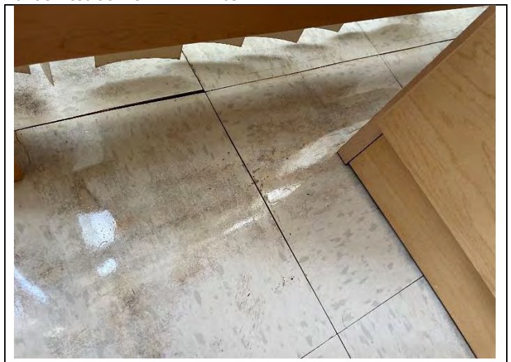
12. View of water damaged floor tiles adjacent to sliding balcony door in PEI 212
