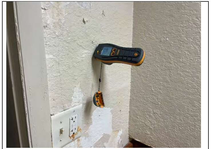
36. View of water damage and elevated moisture levels using Protimeter in restroom walls of PEI 345
