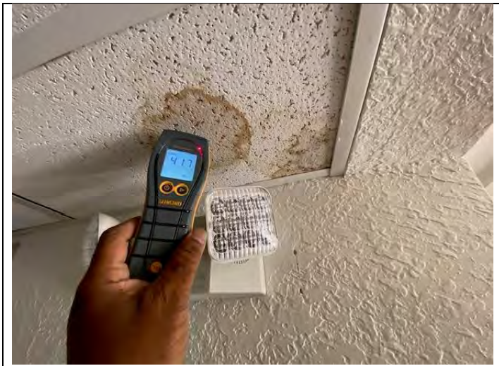
23. View of water damaged ceiling tile with elevated moisture levels using Protimeter in PEI 2 Lounge kitchen
