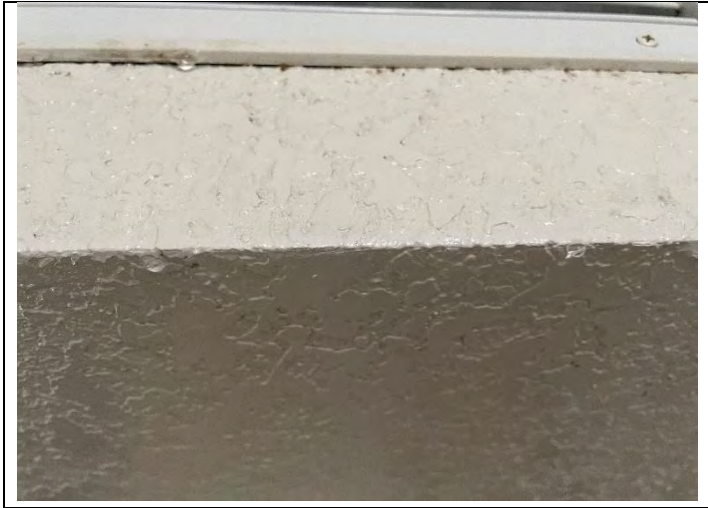
9. Close up view of condensate on supply diffuser in PEI 216
