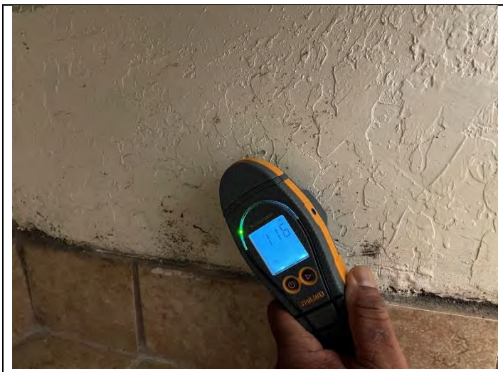
39. View of SVG with dry moisture level with Protimeter under restroom sink in PEI 331
