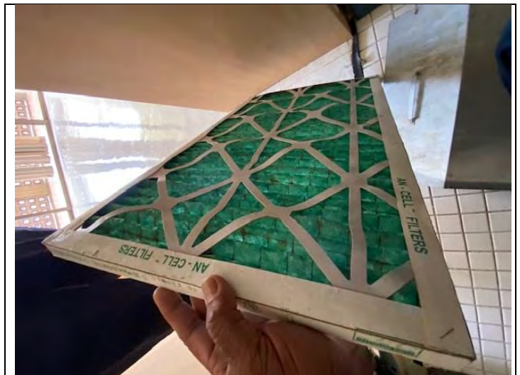
20. View of saturated HVAC filter found in PEI 240
