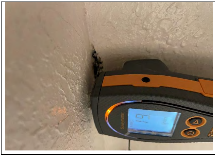
13. View of SVG and elevated moisture levels using Protimeter under restroom sink in PEI 221
