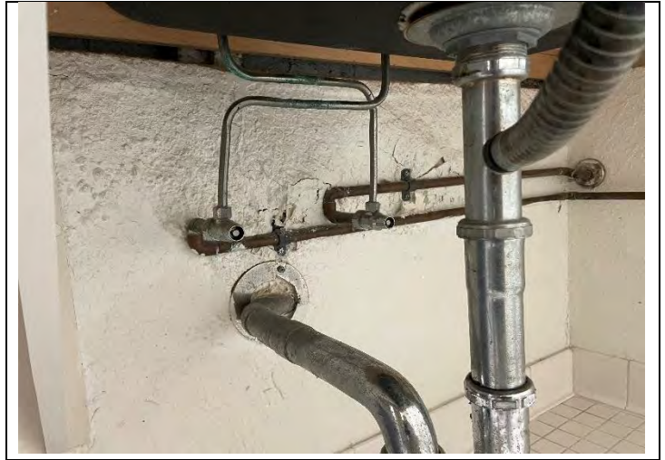
10. View of long term water damage and efflorescence on wall under restroom sink in PEI 205
