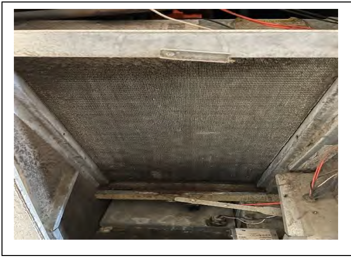
7. Interior view of typical HVAC coil observed in all units
