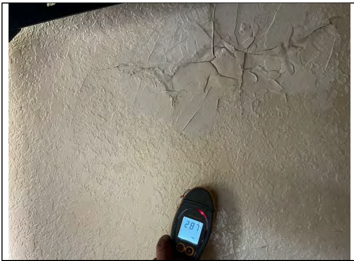
43. View of moisture damage and elevated moisture with Protimeter on North wall in PEI 342
