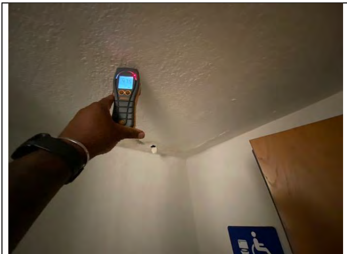
21. View of SVG with elevated moisture levels using a Protimeter on ceiling outside restroom in PEI 2 Lounge
