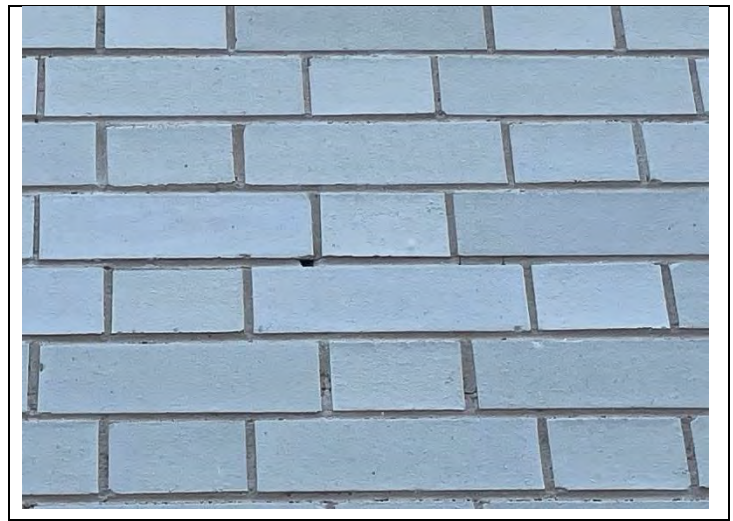
44. View of typical exterior PEI 2 and 3 buildings with identified holes in grout.
