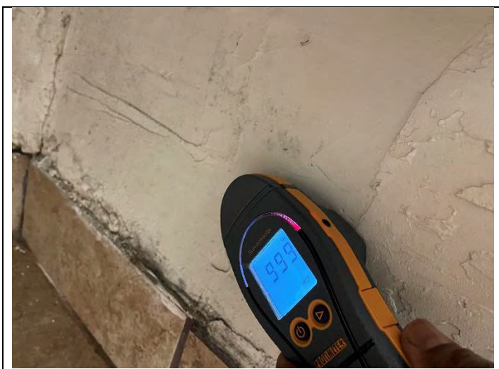
41. View of SVG and elevated moisture level with Protimeter under restroom sink in PEI 308
