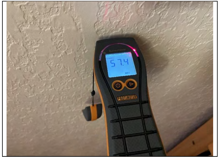
32. View of elevated moisture in ceiling and wall material around HVAC system in PEI 307
